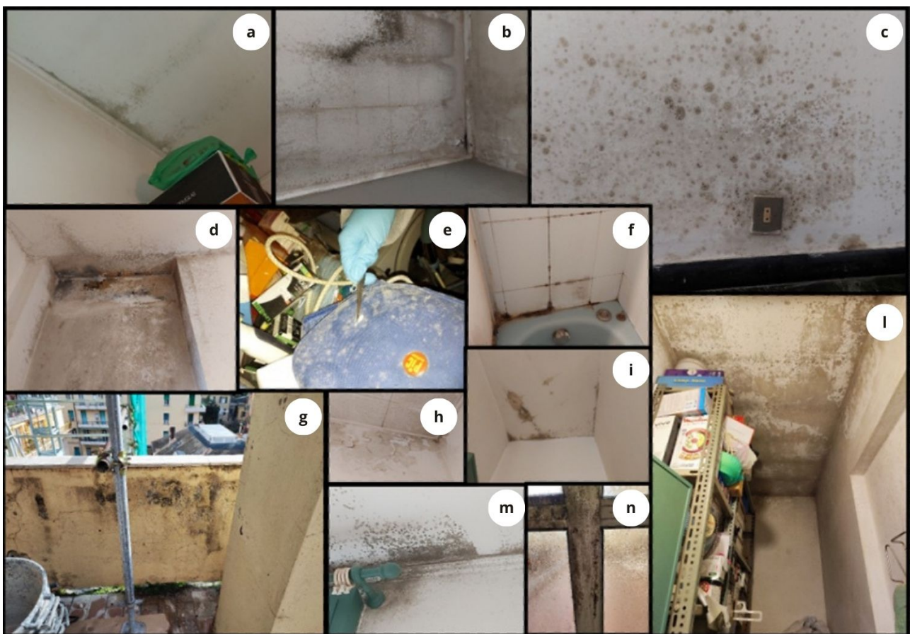
Fig. 1 – Fungal contamination on various surfaces of the apartment: a. entrance ceiling, b. bedroom ceiling, c. living room wall, d. corridor niche, e. items in the pantry, f. bathroom wall, g. terrace, h. bathroom ceiling, i. kitchen ceiling, l. pantry, m. single bedroom ceiling, n. single bedroom window.
